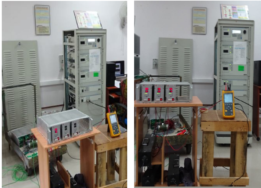
Figure-18: The Power Quality Testing Equipment Connected to ECPS (left showing testing of single ECPS unit, right showing the testing of Multiple ECPS units)
