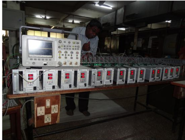
Figure-29: Latest embodiment of ECPS SM100 fourteen of them sharing the load
